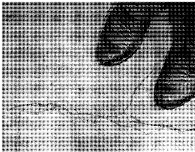
Cracks show: basement floor after a tremor in 2011 — Getty
